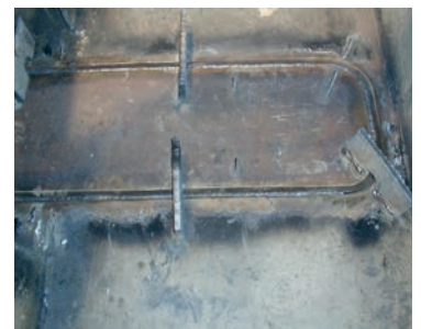
Above: Trial fit of external cofferdam for large insert repair of offshore vessel (main picture). Typical flat insert repair showing single sided weld (top smaller picture) and Insert held in place with 'dogs' (bottom smaller picture).
