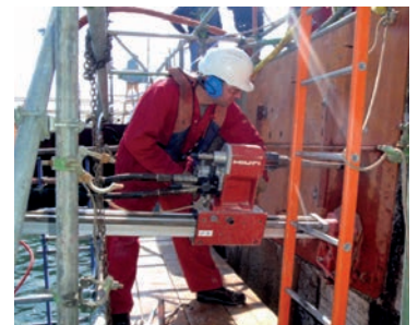
Main image: Revetment levelling and reinforcement on River Thames. Above: Installation of piled concrete plinths (top). Positioning of drilling jigs at Ocean Basin (second). Precision diamond drilling for quayside strengthening (third).
